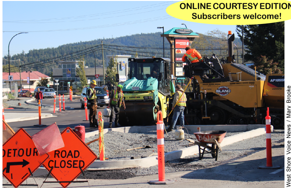
Paving and curb preparation has been actively underway for weeks at Evergreen Shopping Centre in Sooke (this photo October 9). WSV
