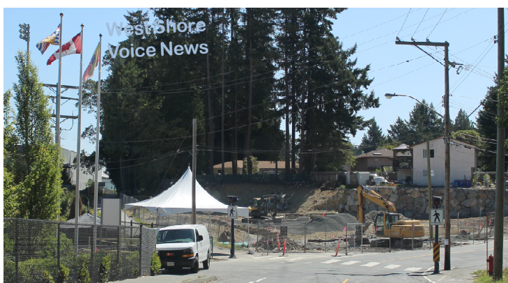
Sarah Beckett Memorial Playground under construction on Glen Lake Road behind Westhills Stadium (July 20, 2019).
