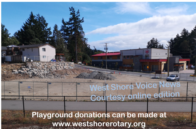
Sarah Beckett Memorial Playground site development continues along Glen Lake Road behind Westhills Stadium (June 23). Rock wall and fencing underway.
