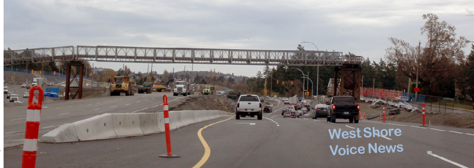
New lane configuration during construction on Highway 1 at the Mackenzie/Admirals interchange (southbound view, November 5) in place until summer 2019.
