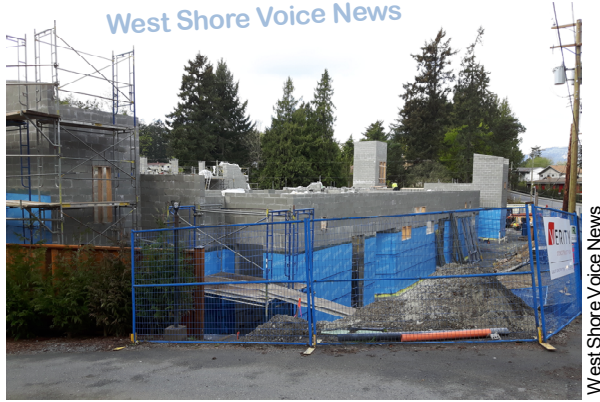
The two-storey 19,000 sqft Rugby Canada high-performance training facility is under construction on about one acre on Glen Lake Road in Langford.
