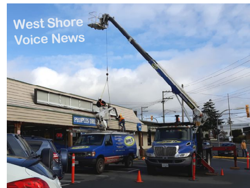
A new PEOPLES overhead sign was installed on November 28, 2016. It will soon be changed to a PHARMASAVE sign.
