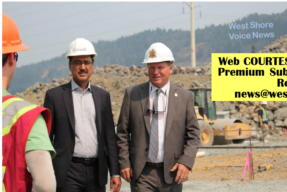
Federal Minister of Infrastructure and Communities Amarjeet Sohi toured the West Shore Parkway construction site with Langford Mayor Stew Young, August 2.
