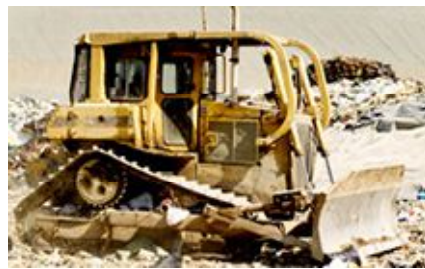
Working the materials at Hartland Landfill. About 114,000 tonnes of municipal solid waste are received at the facility each year. The Capital Regional District projects the current landfill setup being full by 2049.
