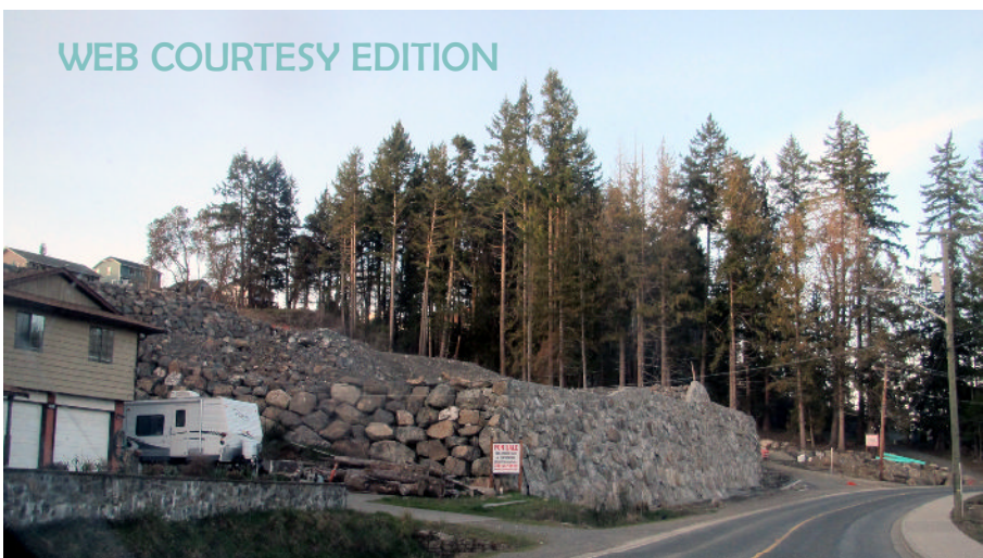
This rock wall along Wishart Road in Colwood is just one of some new retaining wall structures that have generated public complaints to the City of Colwood.
