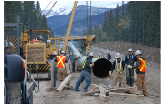
Trans Mountain's Anchor Loop project was completed in 2008 through Jasper National Park and Mount Robson Provincial Park. The project involved installing a second pipeline adjacent to the existing Trans Mountain pipeline between Hinton, Alberta and Hargreaves, BC.
